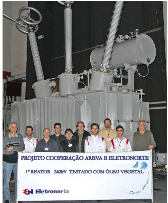
Picture: 242 kV 22 MVA r shunt reactor filled with natural ester oil for major Brazilian utility Electronorte
