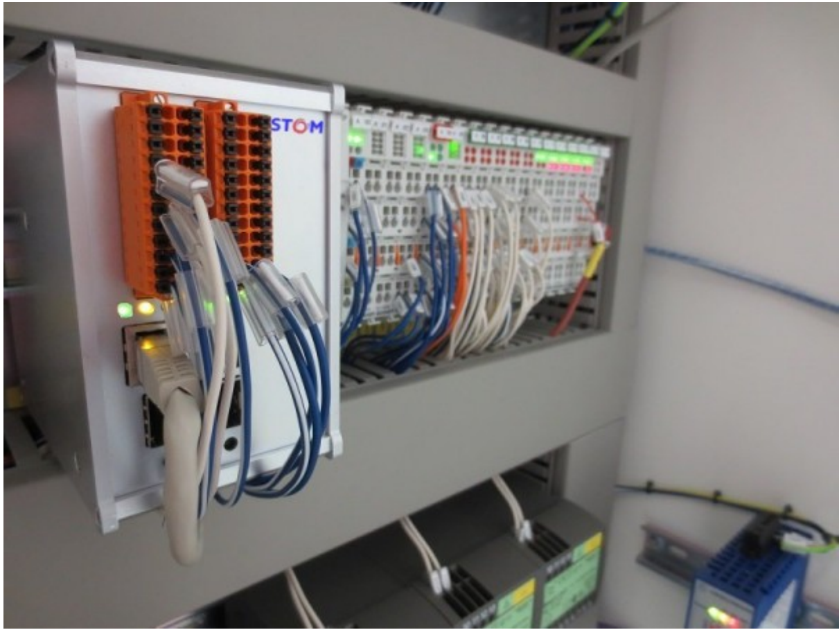
iDAU installed in MS 3000 cubicle
