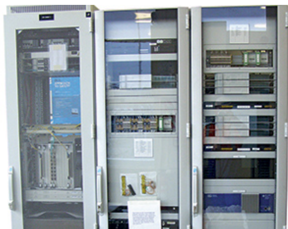
Islington HMI cubicles at the Christchurch substation.
