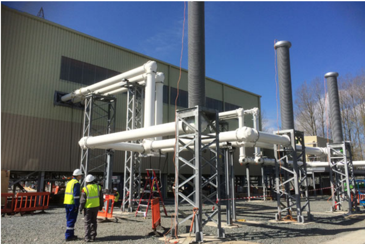
Gas-insulated line project with g 3 at Sellindge UK
